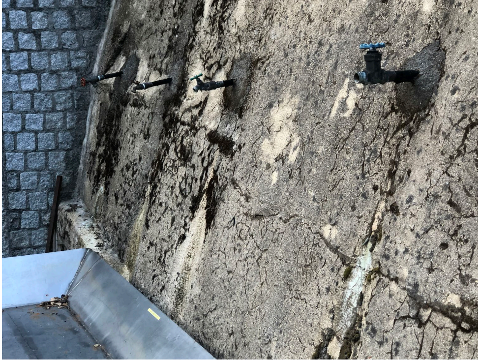
Figure 14. Graywater infrastructure. Spigots from separate garden terraces.
